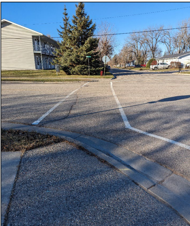
Barrette St./3rd St. NE Intersection - View Showing Apartment Building, Lack of Pedestrian Ramp & Lack of Sidewalk/Street Signage
